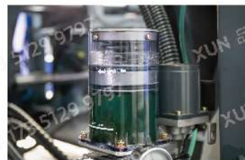
润滑系统 Lubrication oil pump system
